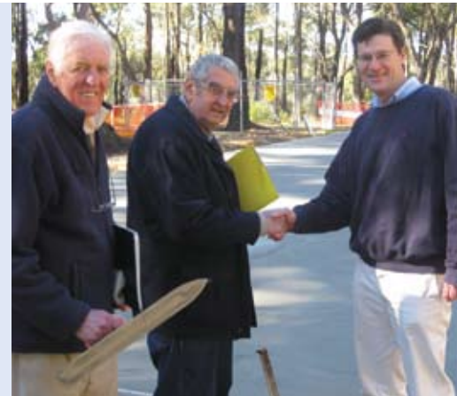
L-R: 'Shed' Vice President Barry Eastment, President Kevin Callinan and Jonathan O'Dea following pouring of the slab.
